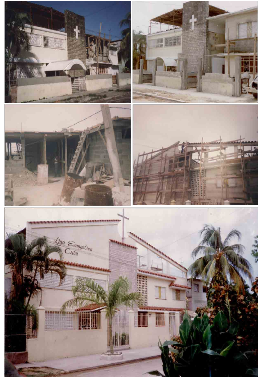
Beginning the 1990s the church experienced massive growth in its membership. The original temple became insufficient, and a series of structural modifications were necessary.
